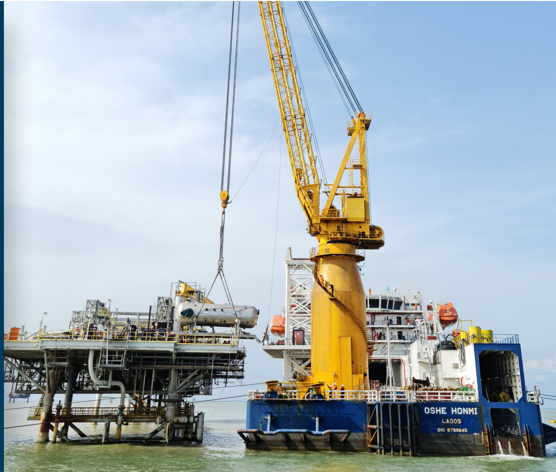
Chevron Okan PRP Platform OML 91, Escravos Area, offshore Nigeria
