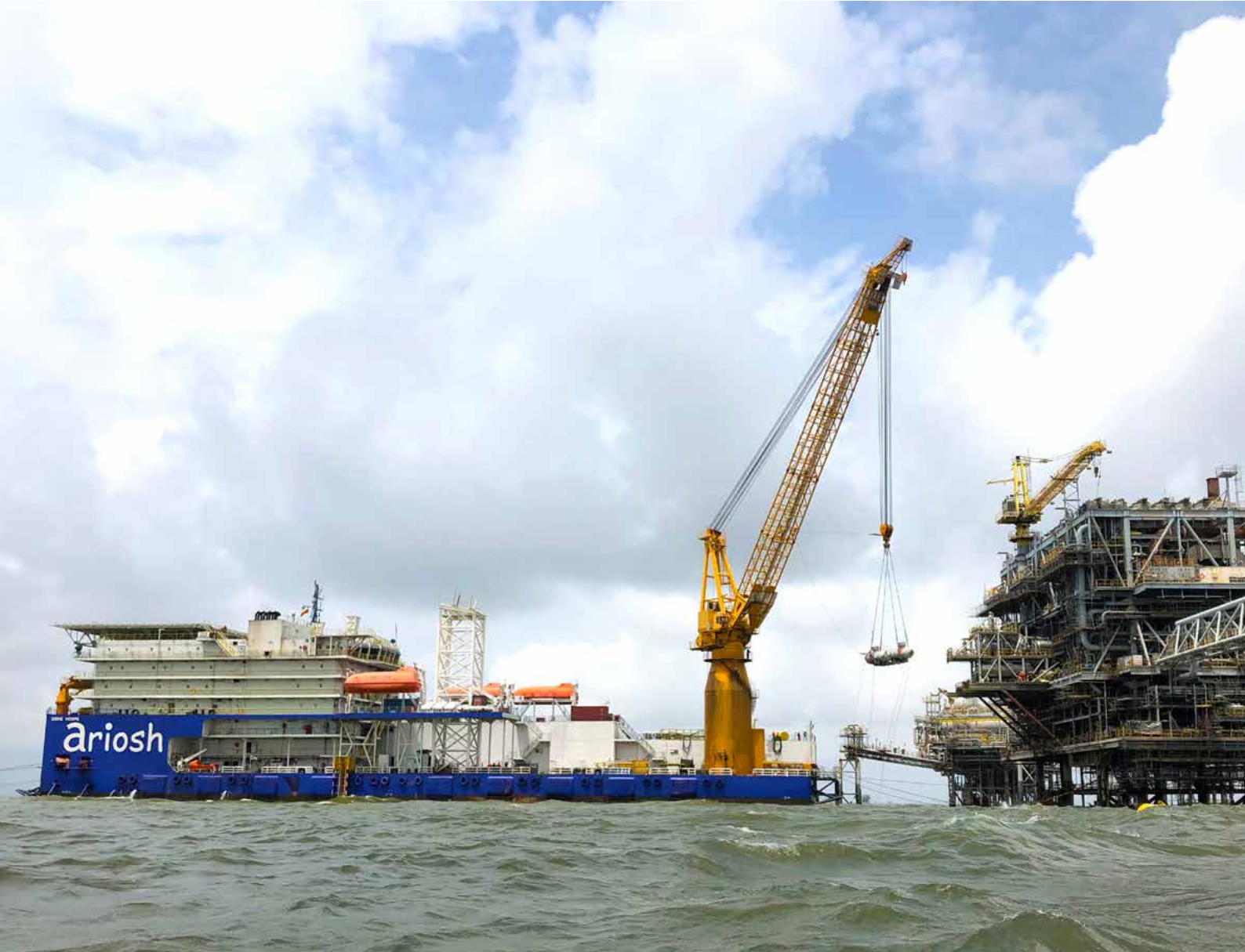
Chevron Okan GGCP Platform OML 91, Escravos Area, offshore Nigeria
