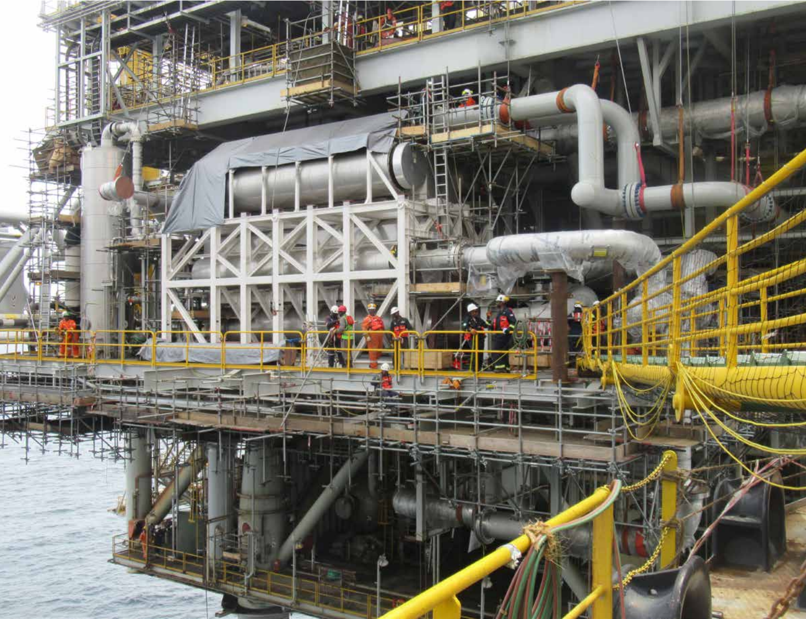
Exxonmobil EAP GX Platform offshore Nigeria
