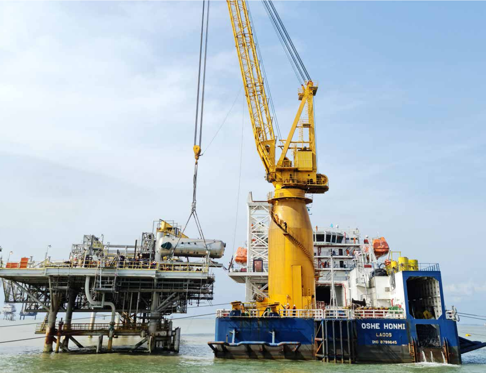
Chevron Okan PRP Platform OML 91, Escravos Area, offshore Nigeria
